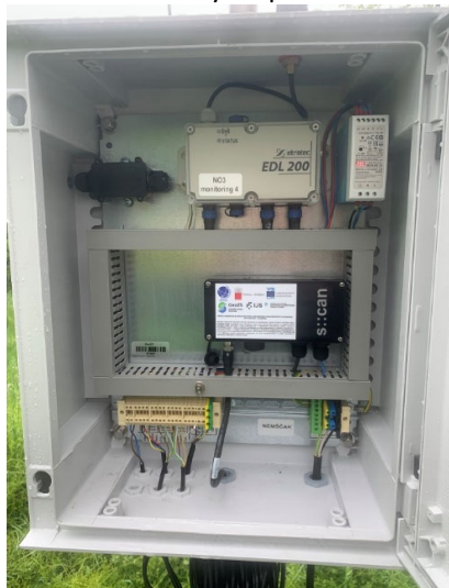
Control unit in a protective box.
