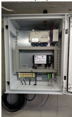
Control unit in a protective box.
