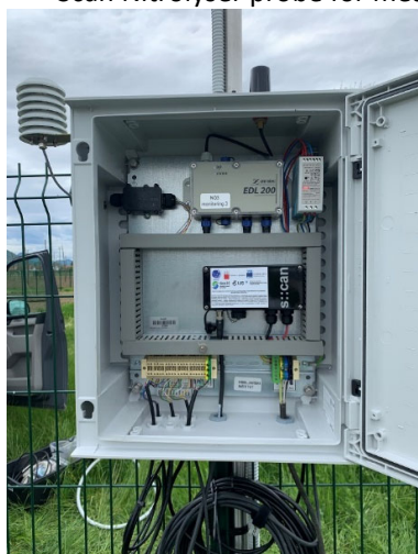
Control unit in a protective box.
